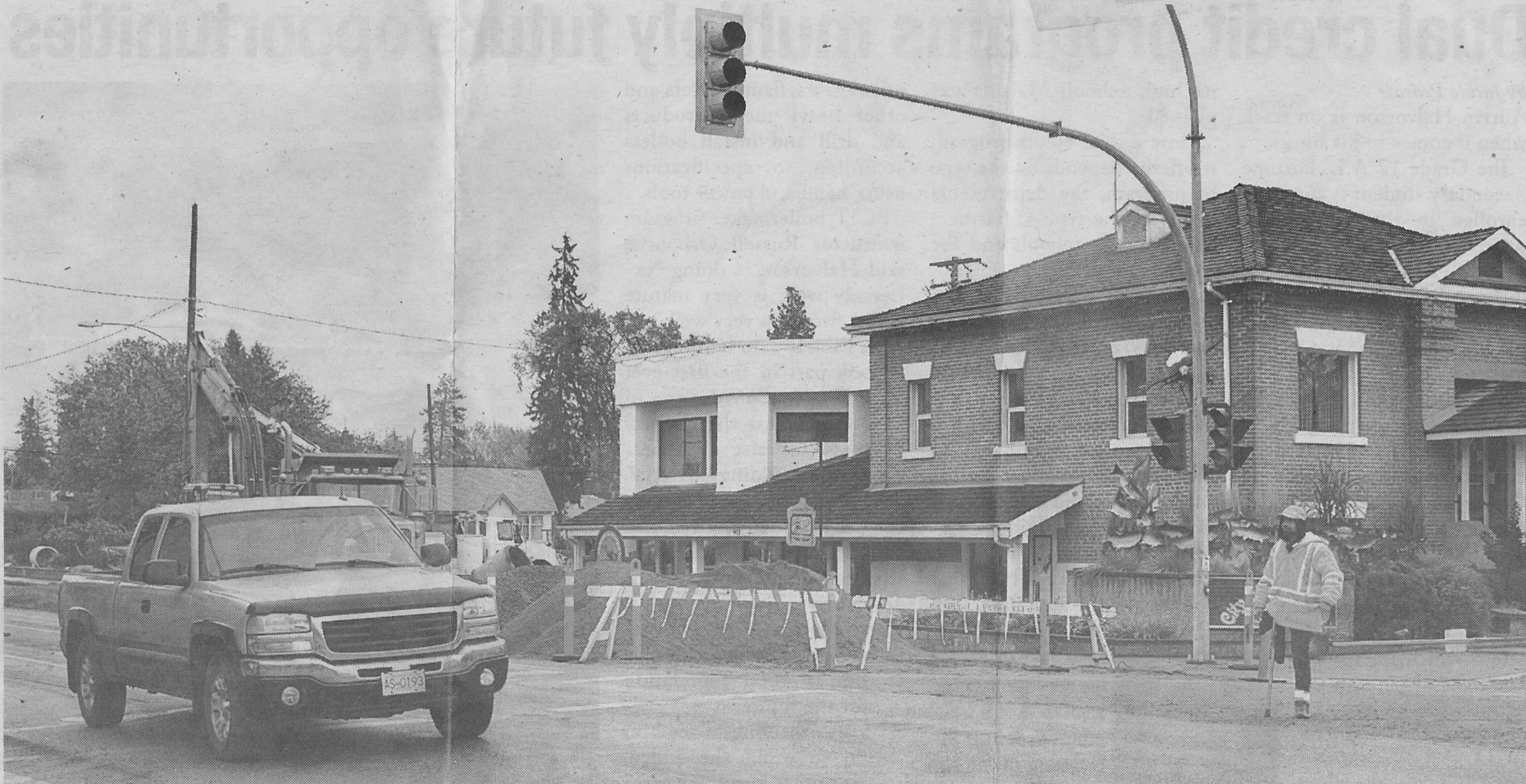
Construction confusion. Flaggers are at the intersection of Cliff Avenue and the highway to direct traffic and pedestrians during construction. The work will close the intersection this week.
